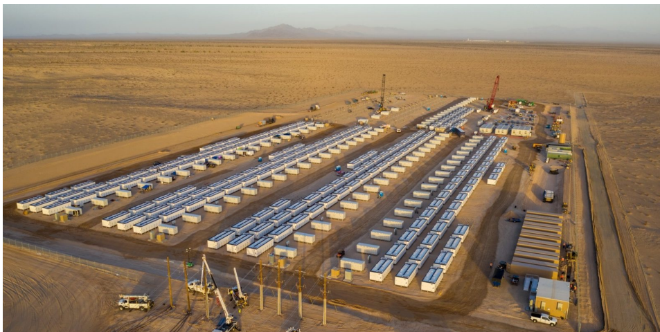
Crimson Storate - 350 MW / 1400 MWh battery storage, California
